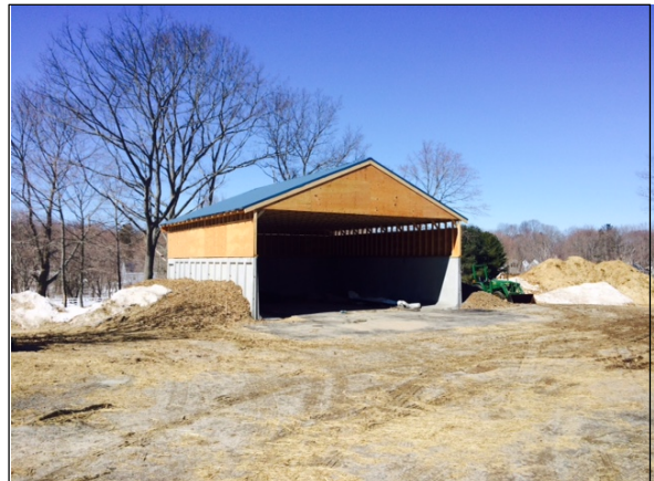
A covered manure storage facility was built at Walnut Hill Equestrian Center to prevent horse manure from washing into Trout Brook.
