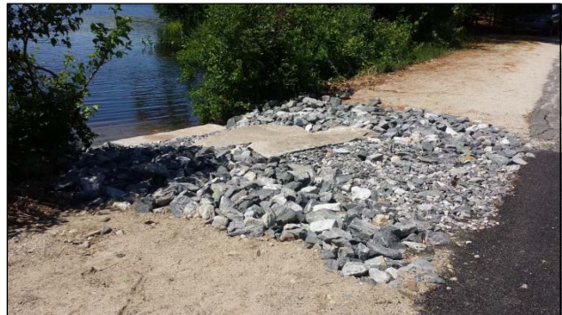
Heath Rd. Boat Launch (After) – Split face blocks were installed in a terraced manner. Stone riprap and geotextile were placed around the blocks to support the road shoulder and pavement edge.
