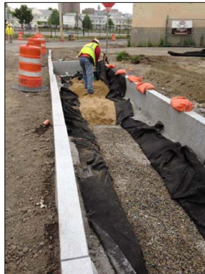
Biofilter installed in Portland in 2016 using CWSRF
