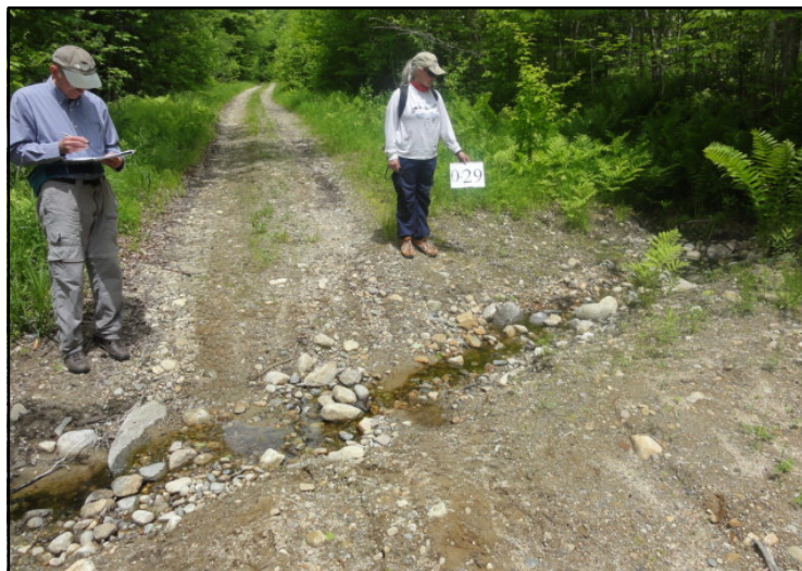
The Ellis Pond Phase I project plans to address 52 of the 183 erosion sites identified during their 2014 watershed survey.
