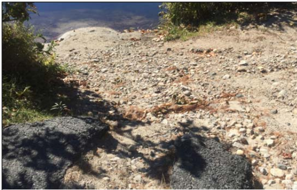
Heath Road Boat Launch (Before) – This site was severely eroded due to heavy use as an unofficial boat launch and snowmobile access
