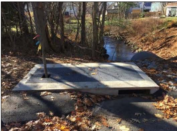
A StormTree system was installed to treat 0.5 acres of impervious area. An educational sign will be placed at the site to explain the BMP function.
